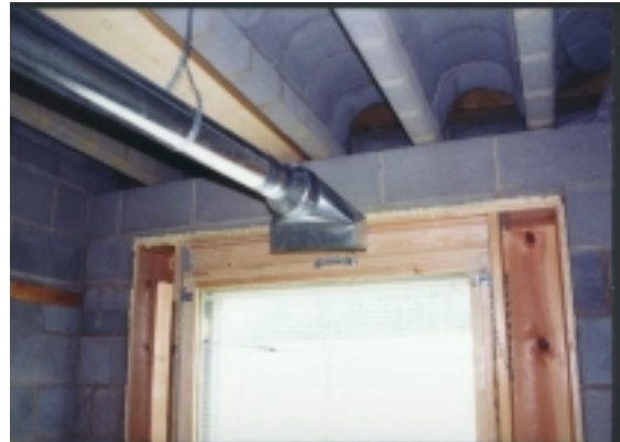
Fig 4.18 Returning air intake
