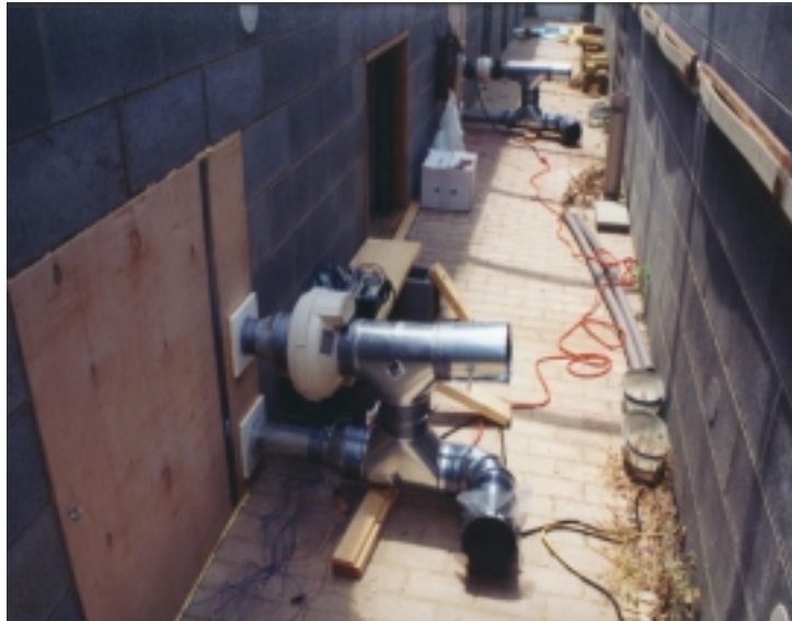
Figure 4.9 The ventilation fans at the rear corridor
