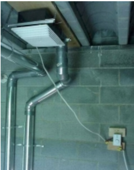
Figure 4.8 Ceiling Fan and Heater and Thermostat
